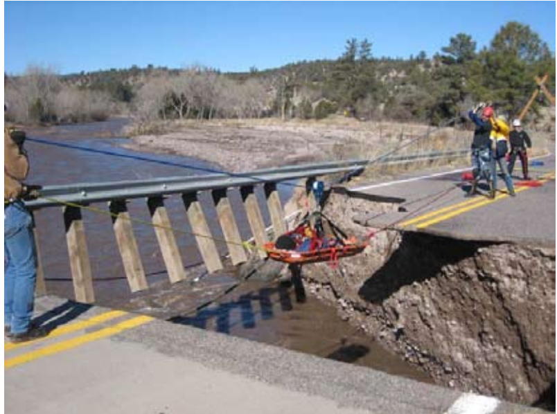
New Mexico Search and Rescue crews and local fire crews whisk Georgene Fritz across the 18-foot gap of the North Fork Bridge near the Gila Cliff Dwellings Tuesday. The bridge was washed out by flash flood waters caused by rains and warm temperatures Sunday night. (Photo for the Sun-News by Fred Potter)
